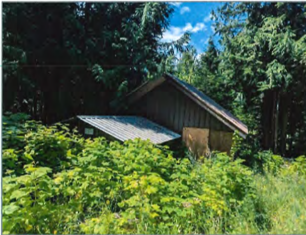
Photo 1. Powerhouse within 30 m WDP area (July 7, 2026).
