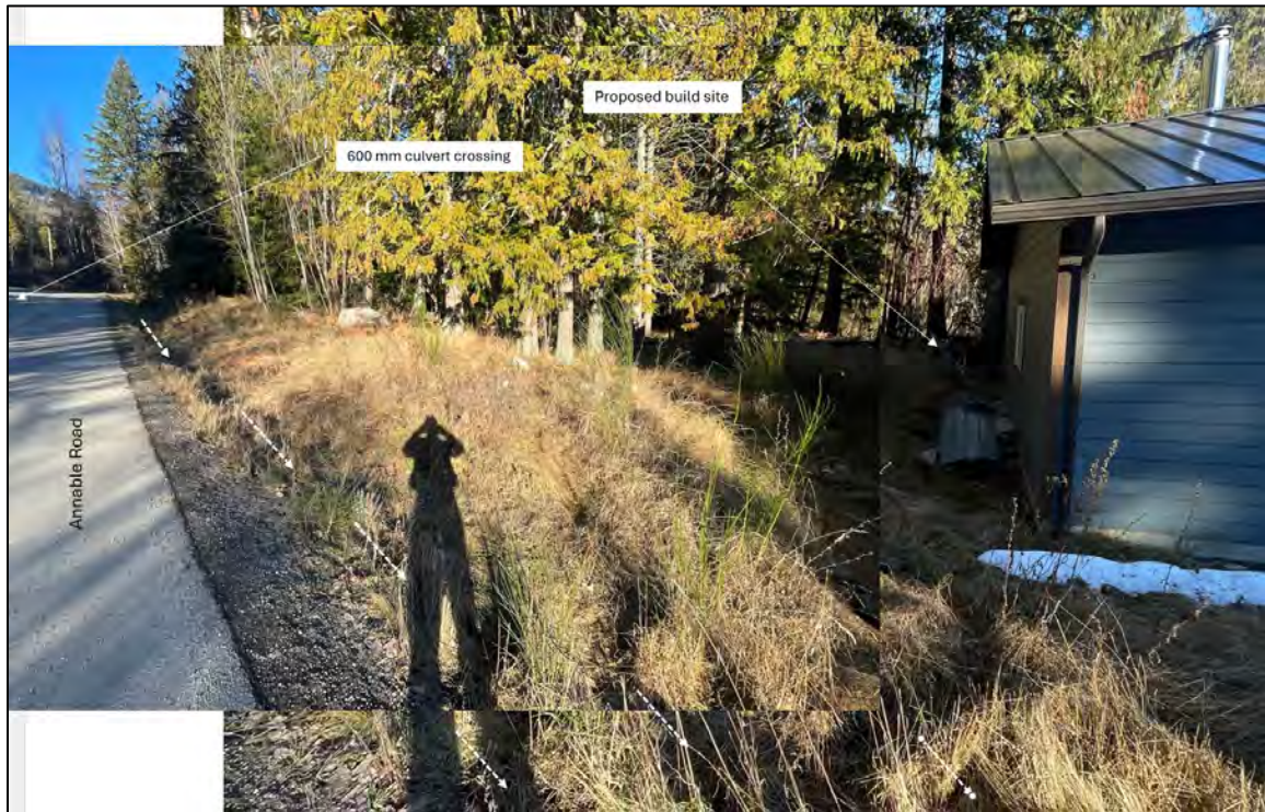
Photo 7: View looking at the Annable Road surface and ditch adjacent to the property. The white flow directional arrows indicate the path of overland flow from a blockage/ capacity exceedance at the 600 mm culvert crossing on Annable Road.
