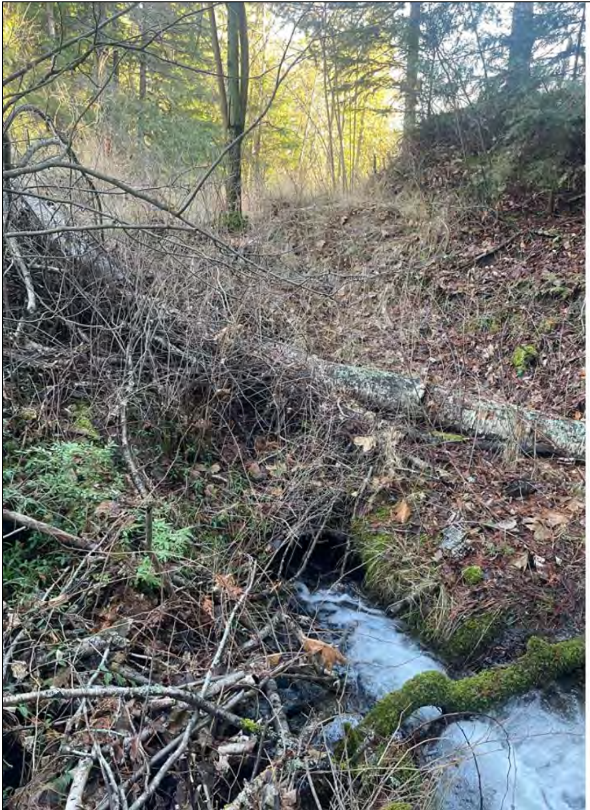
Photo 3: View of entrance to 600 mm diameter culvert under Annable Rd crossing at on north end of the property approximately 60 m upstream from the proposed build site.
