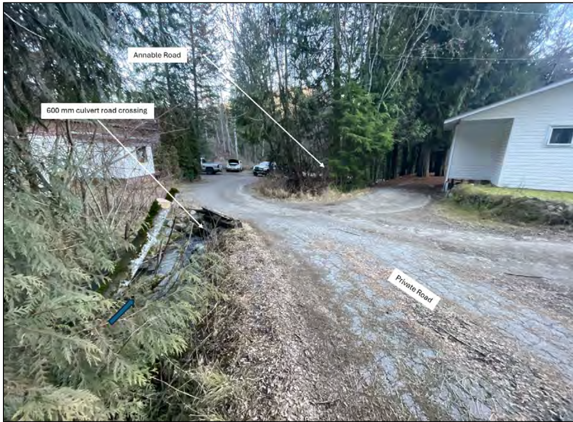
Photo 5: View showing culvert road crossing on private road approximately 30 m upstream from the 600 mm culvert crossing at Annable Road shown in Photo 3.
