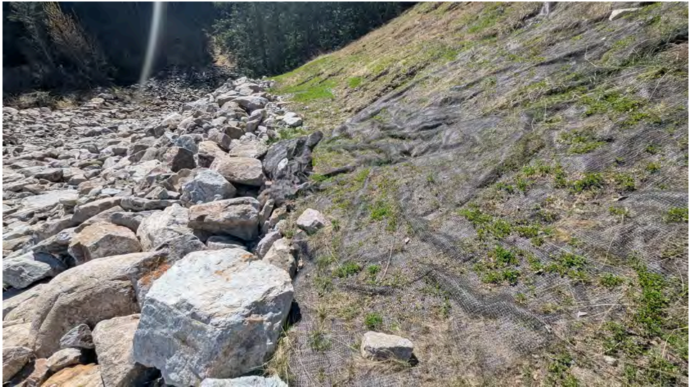
Photo 18: Right bank of the spillway looking downstream showing the area repaired in 2023. The repair is in good condition with no signs of instability.
