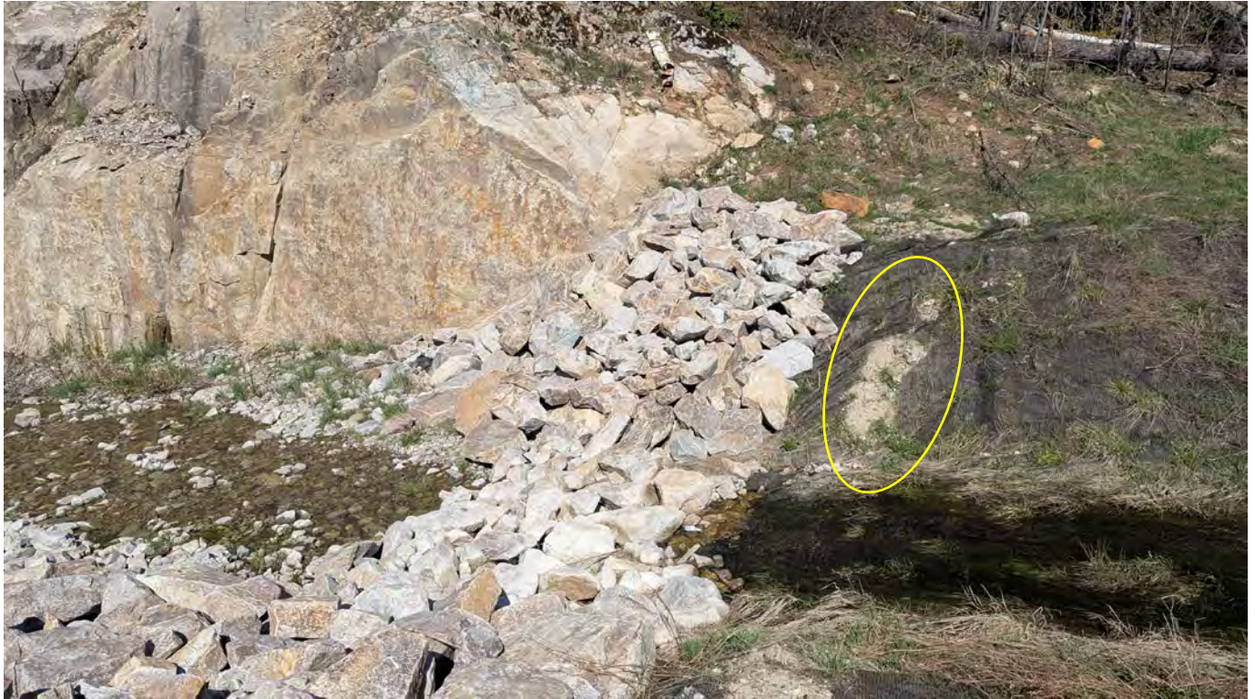
Photo 11: Riprap at the spillway inlet. The sand material upstream of the inlet (circled) is overtop the Turf Reinforcement Mat (TRM) and is not a tear of the TRM. Sand was likely deposited during the riprap placement in 2023.
