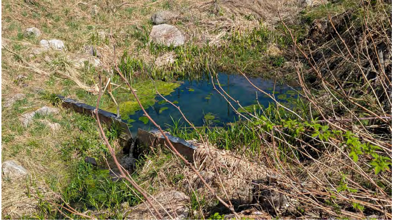
Photo 20: V-notch seepage weir. Seepage was clear with no signs of sediment deposition..
