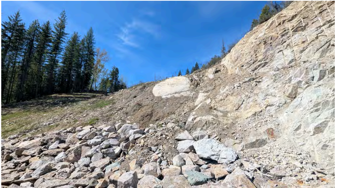
Photo 16: Erosion gully at the downstream end of the bedrock highwall adjacent to the spillway. The gully is self-armouring and the conditions are unchanged compared to the 2024 inspection.
