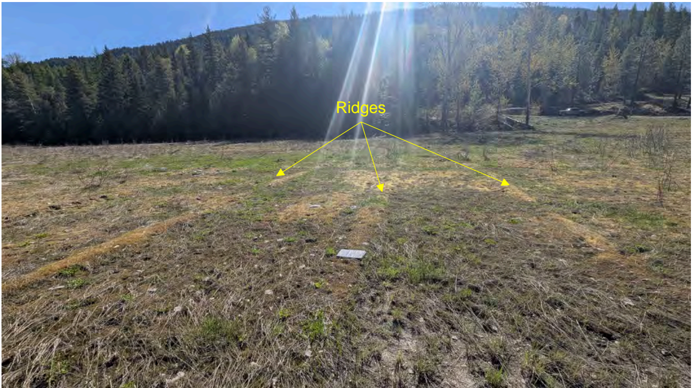
Photo 4: Small ridges are present in the tailings pond backfill area that are about 10 cm high and spaced 3.0-3.5 m apart. Ridges are suspected to be located where the Combigrid overlaps occur from the 2021-2022 construction.
