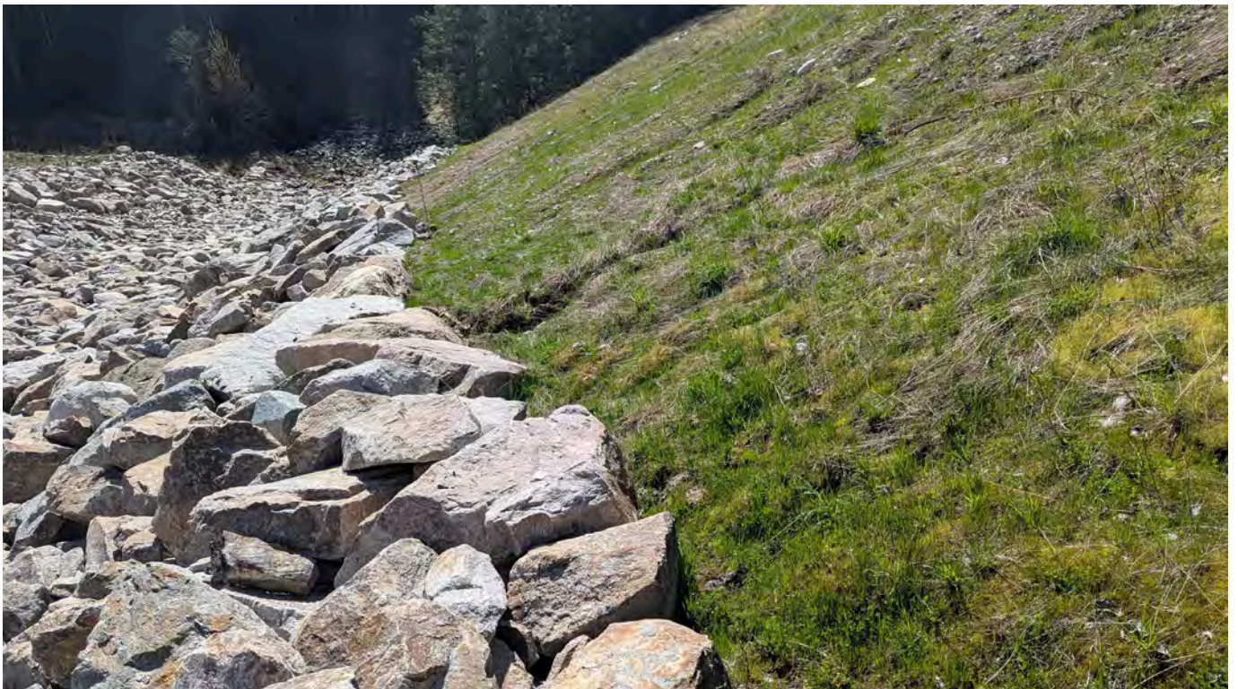
Photo 17: Right bank of the spillway looking downstream. A small erosion gully is present. Any water flowing down the gully flows overtop the geotextile and into the spillway. No actions are required.
