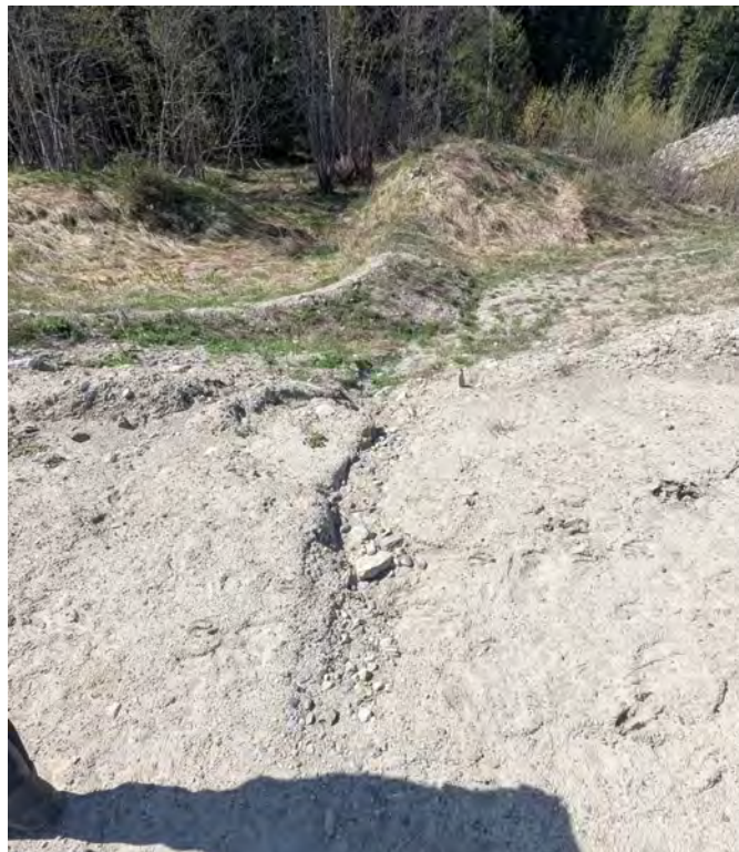
Photo 27: Erosion gully in the toe berm crest near the east abutment. Due to concentrated flow from the toe berm crest.
