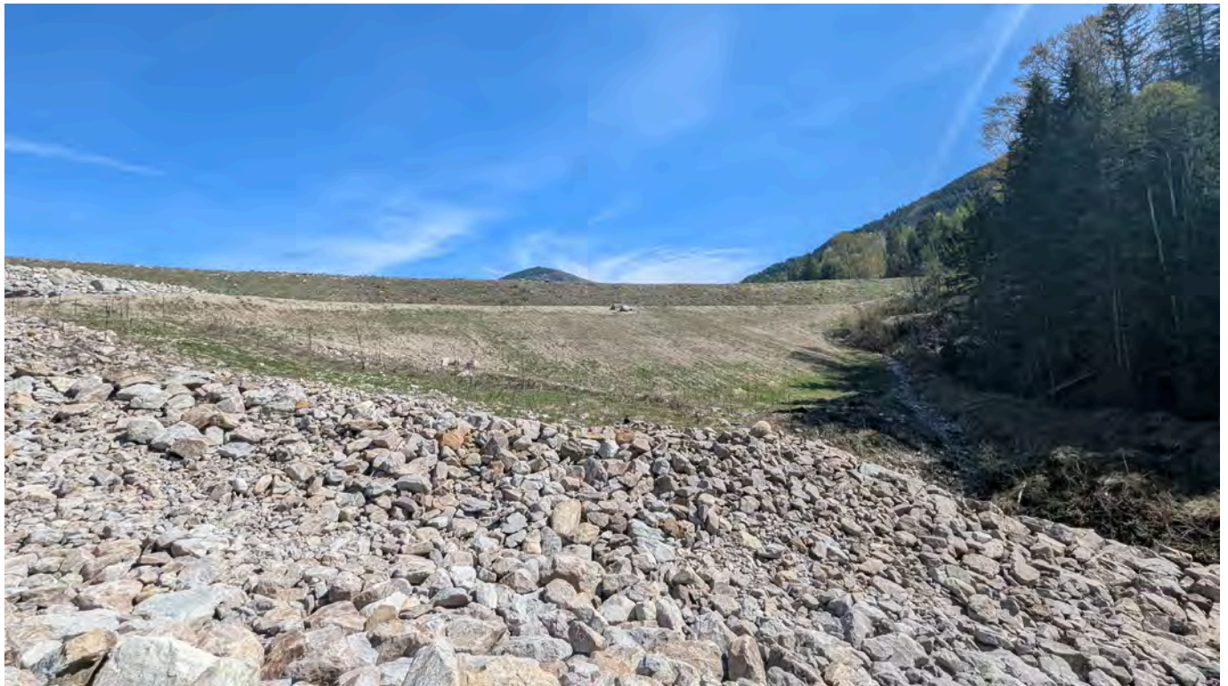
Photo 19: Downstream slope of the dam and left bank of the spillway looking north.
