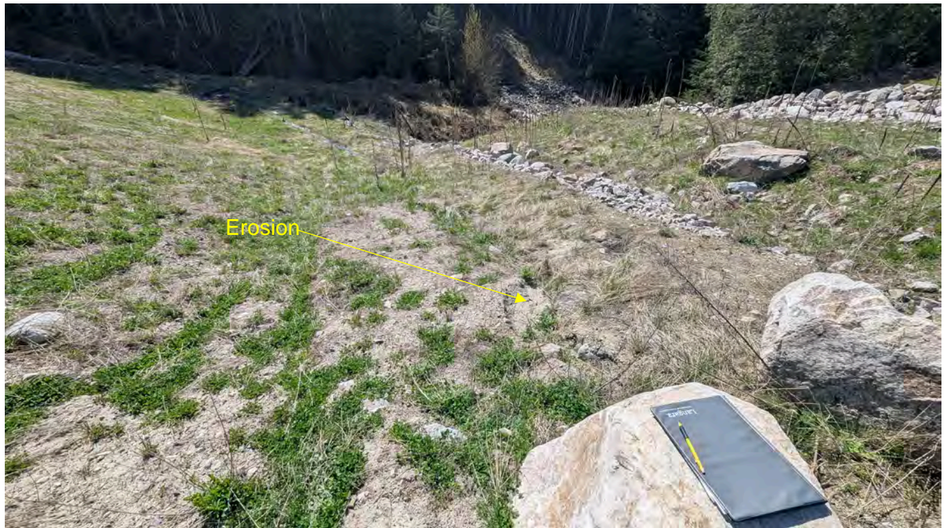
Photo 23: Downstream slope of the toe berm at the west abutment looking downslope from Piezometer P3. A small erosion gully is present orientated parallel to the slope approximately 5 cm deep, 5 cm wide. Continue to monitor.
