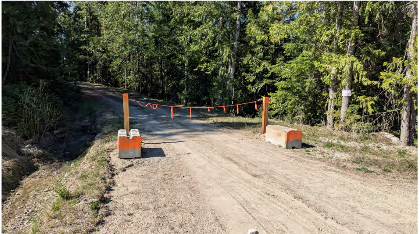
Photo 1: New gate installed on the road from the Central Landfill to the HB Dam to restrict access.
