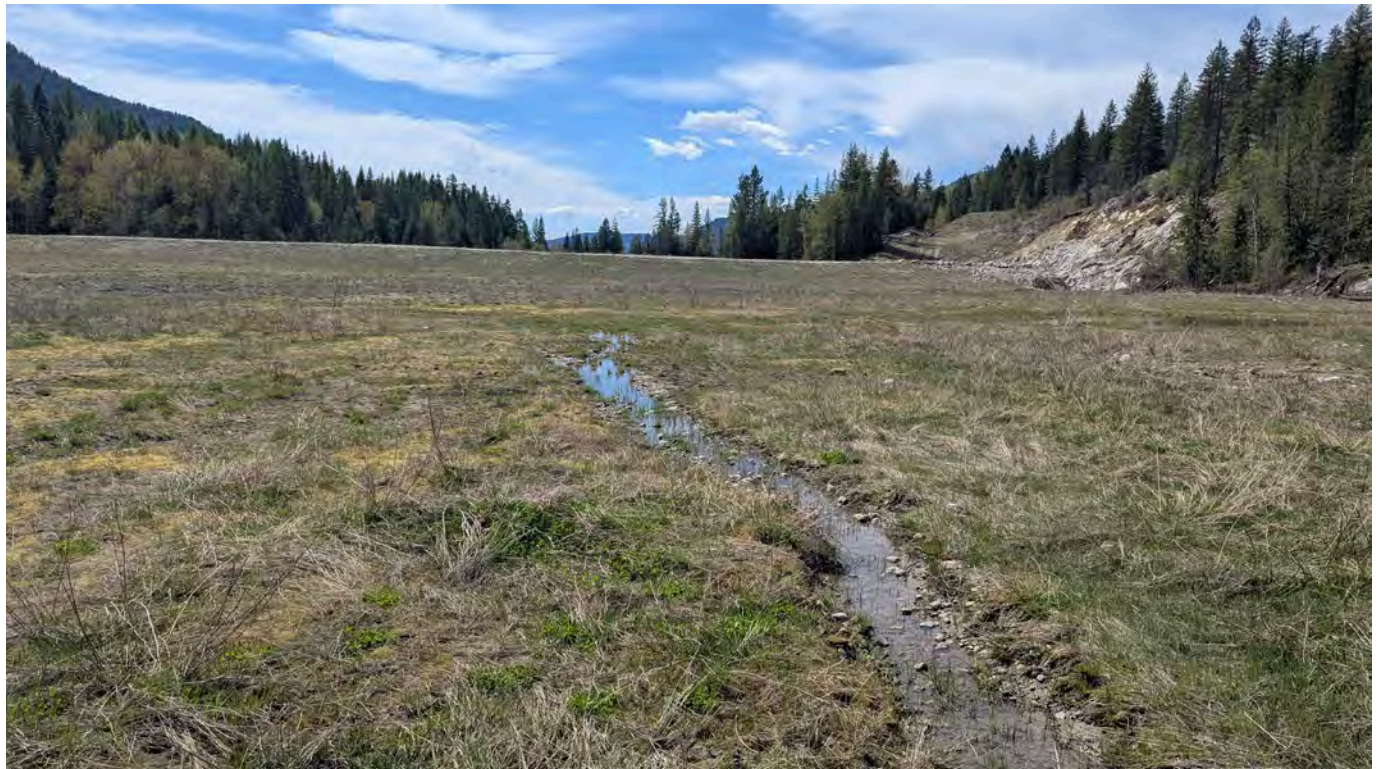
Photo 32: Small channel formed from runoff on the west side of the TSF looking south. Water flows parallel to the Main Channel and enters the Main channel near the spillway. No change compared to the 2024 inspection.
