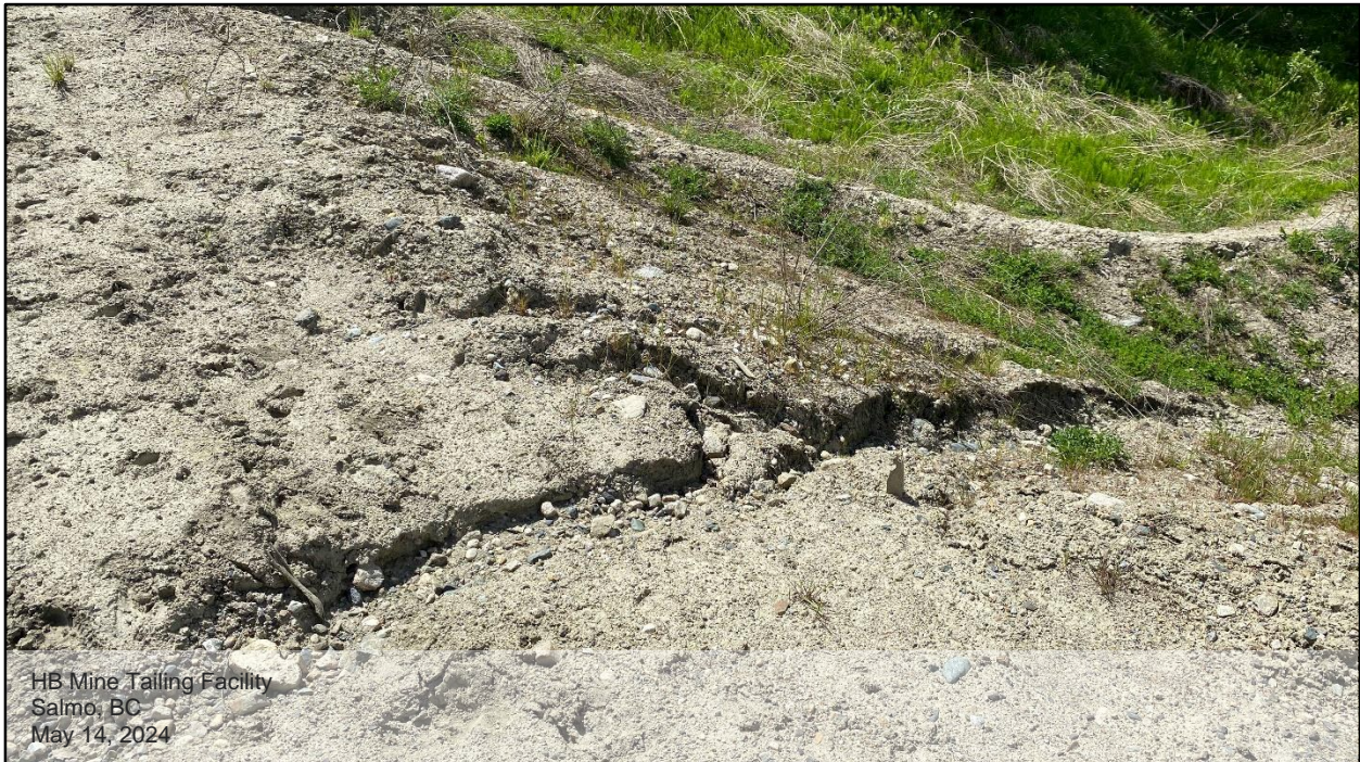
Photo D.23: A close view of the downstream east slope of the expanded berm. The downstream eastern slope of the extended berm is prone to surface erosion and sloughing.
