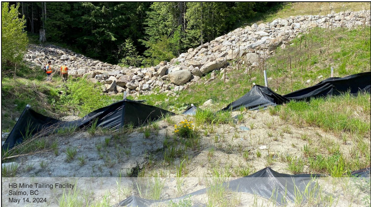
Photo D.16: View of the downstream slope of the expanded berm and toe of the dam, looking south. A sediment control fence was found near the downstream toe. The sediment fence failed at some points and has been covered by sedimented material.
