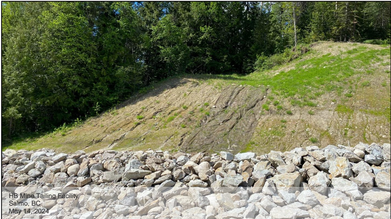
Photo D.15: View of the western slope (exposed till) of the spillway outlet channel, looking west. Surface erosion rills/gullies were observed in multiple locations on the western slope the spillway outlet channel.
