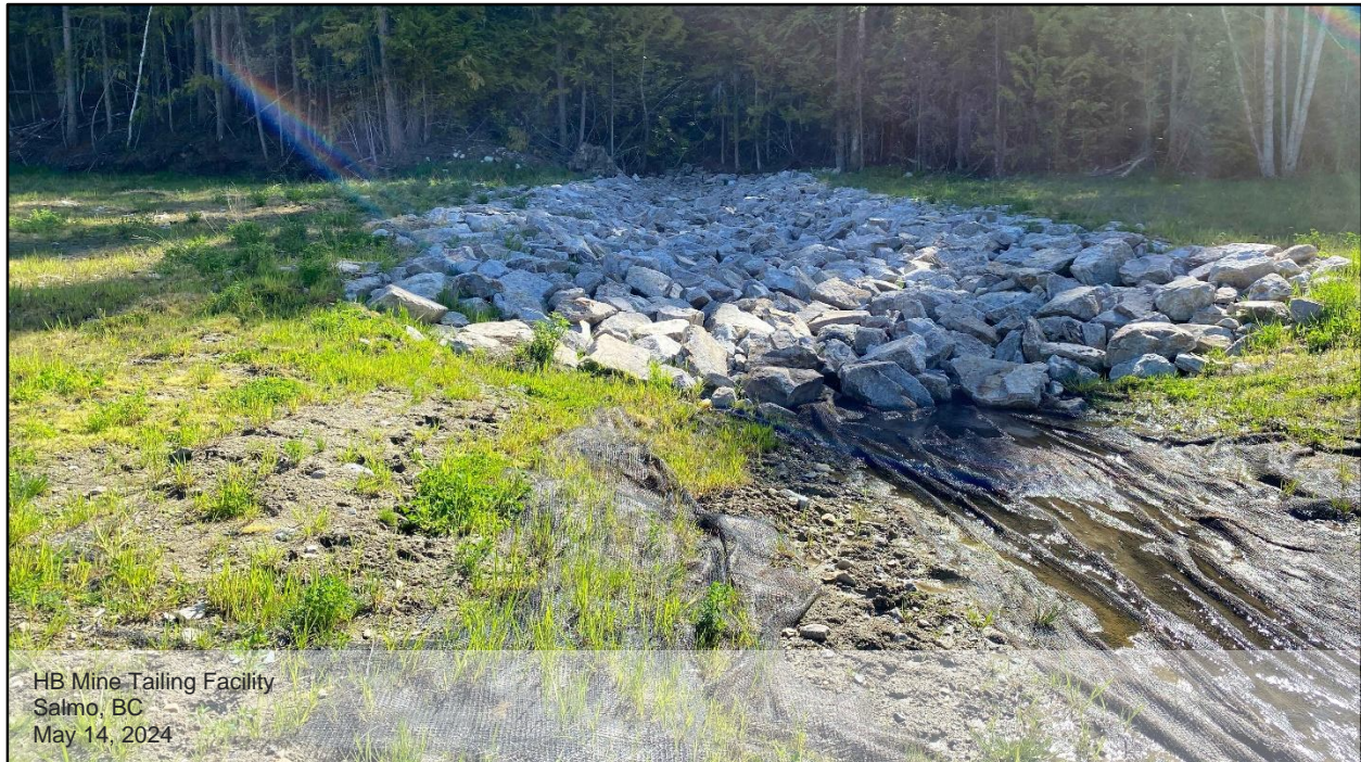
Photo D.29: View of the South Spur Channel inlet and Energy Dissipation Structure (SSCED), looking east.
