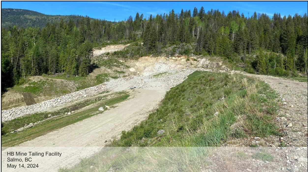
Photo D.5: View of downstream slope face of the dam and the crest of expanded toe berm, looking from the dam crest to west. Well established vegetation was found throughout the downstream slope face.
