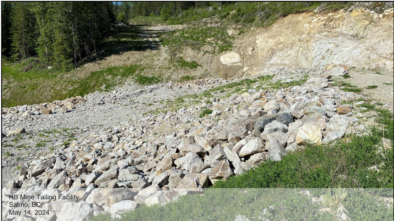
Photo D.9: View of the downstream slope west side, looking southwest. The west side of the downstream slope was repaired in 2012 and a layer of riprap has been placed over this area.
