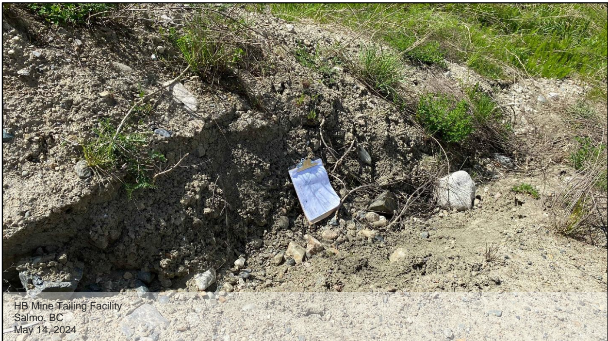
Photo D.24: A close view of the downstream east slope of the expanded berm. Gullies have been developed considerably near the east abutment of the dam.
