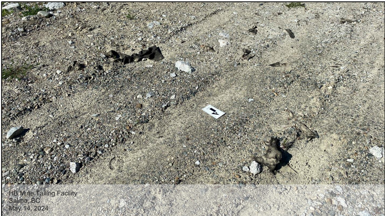
Photo D.10: A close view of the dam crest, west side. Exposed geotextile was observed in multiple locations on the west side.
