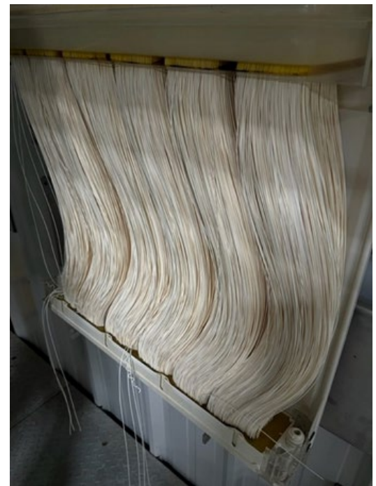
Figure 3-1 Membrane Filter at Arrow Water Treatment Plant
