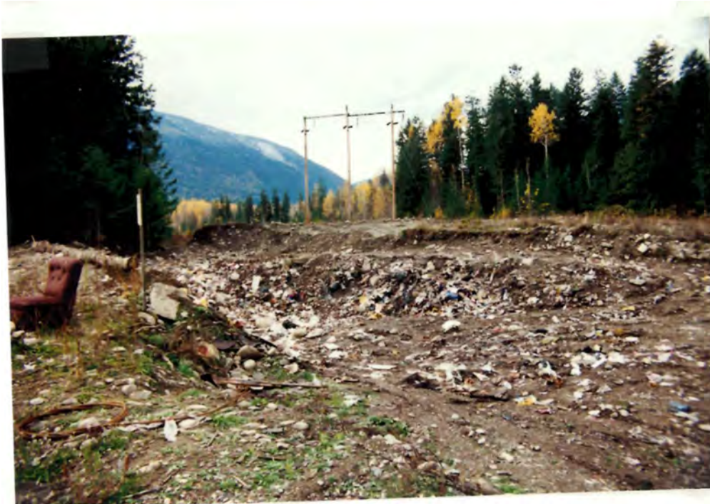
Figure 3: Photo showing trench and fill operation within power line area at the Burton Landfill site. ENV records show photo was taken in November of 1994.
