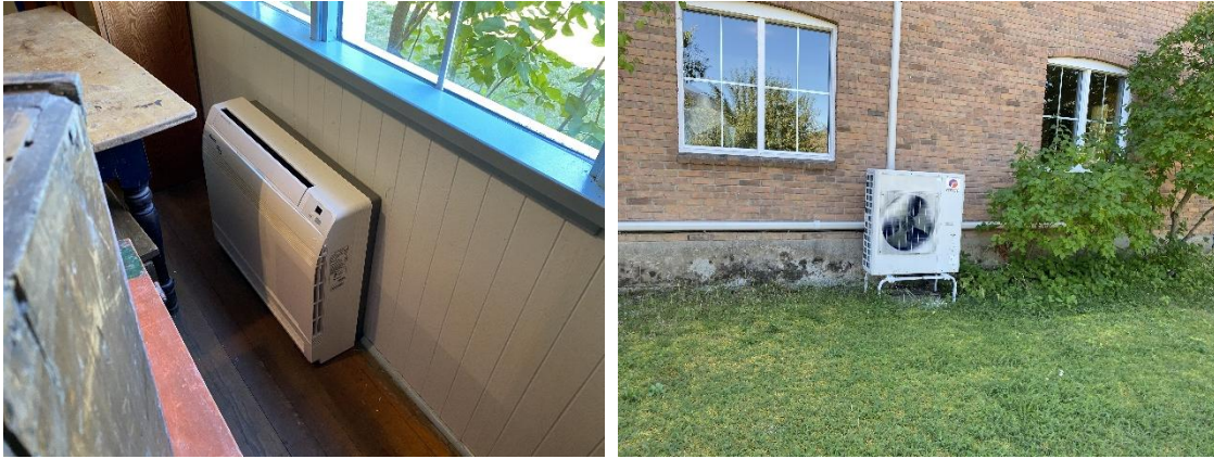
Figure 14: Typical Indoor ASHP Unit and Multi-Zone Outdoor ASHP
