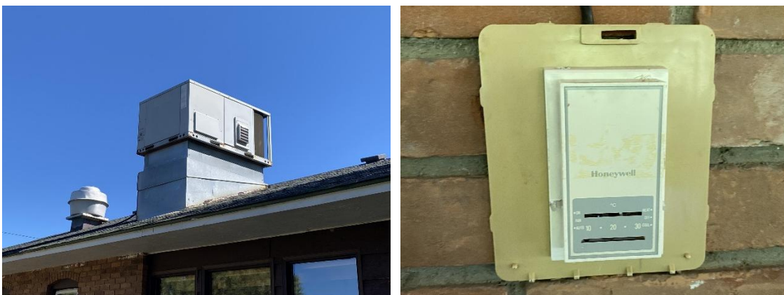
Figure 12: Packaged Rooftop Unit and Non-Programmable Thermostat
