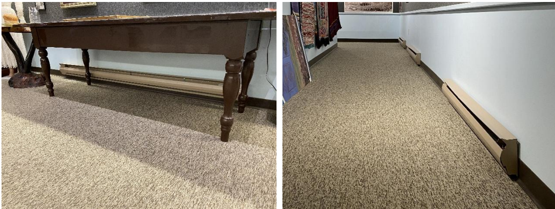
Figure 8: Typical Electric Baseboard Heaters
