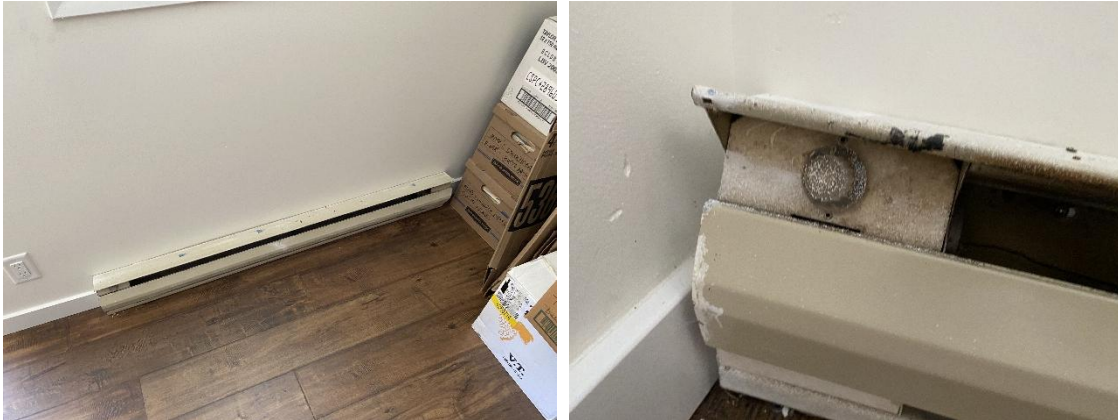
Figure 4: Typical Electric Baseboard Heater and Integrated Control Dial
