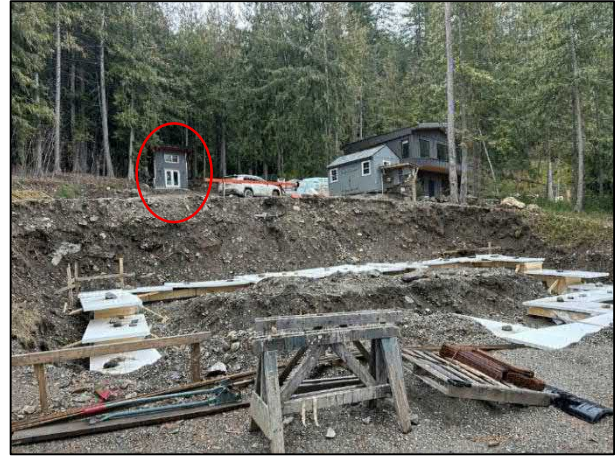
Photo 8. Excavation site with footings for future house and small shed at the back on the left of photo (Feb. 27, 2026).
