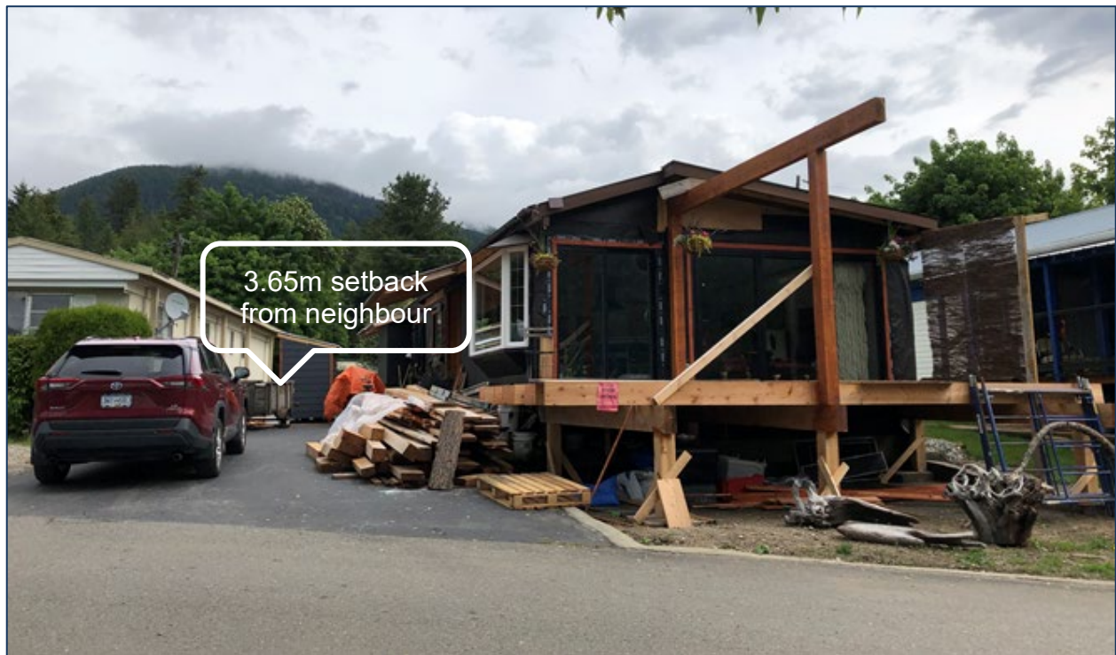
Figure 6: View of property as seen from south-west, showing separation between subject manufactured home and neighbour
