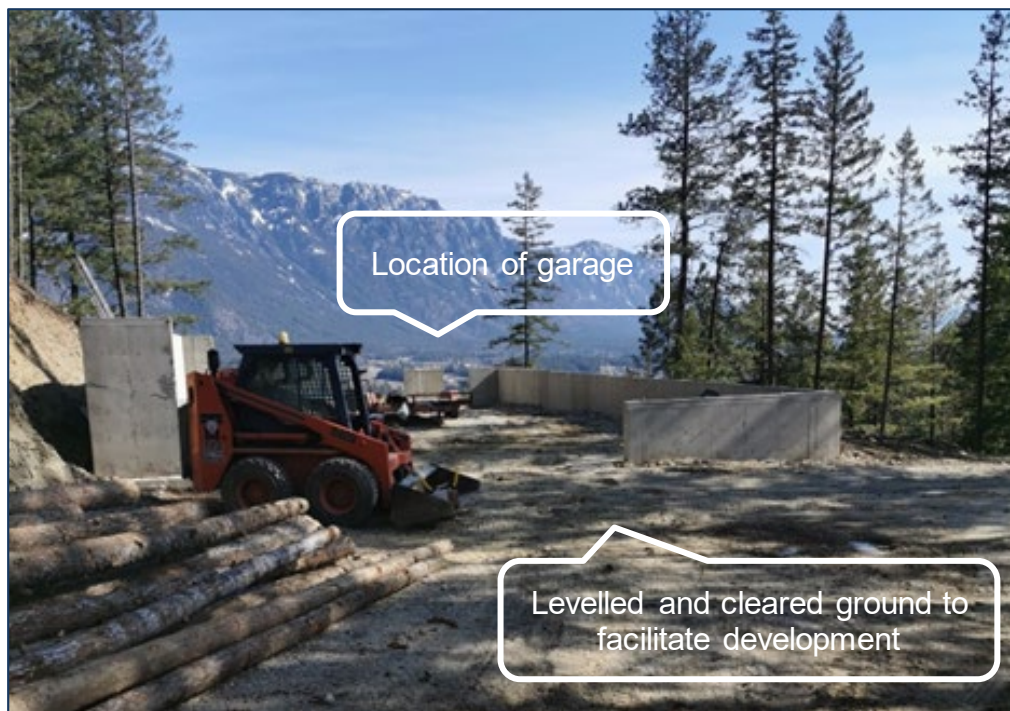
Figure 6: Location of garage as seen from west and facing east. The ground has been levelled and cleared of trees to facilitate the development
