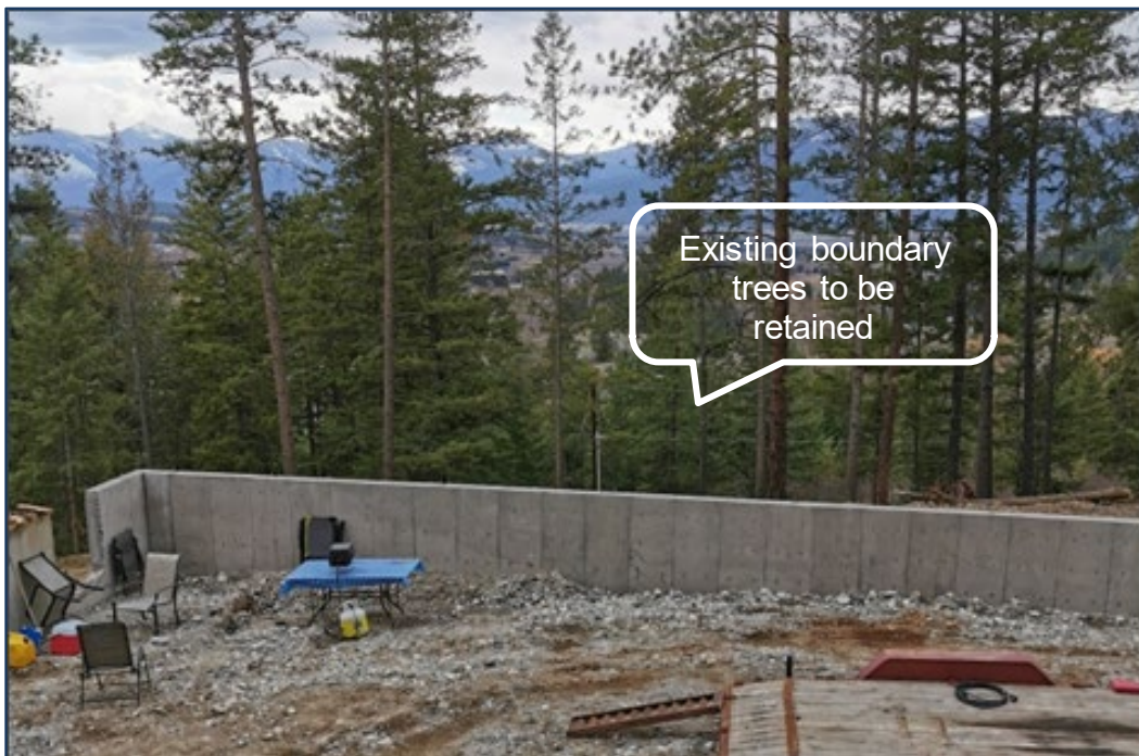
Figure 8: View of existing boundary trees along south-western property boundary, to be retained as part of the development
