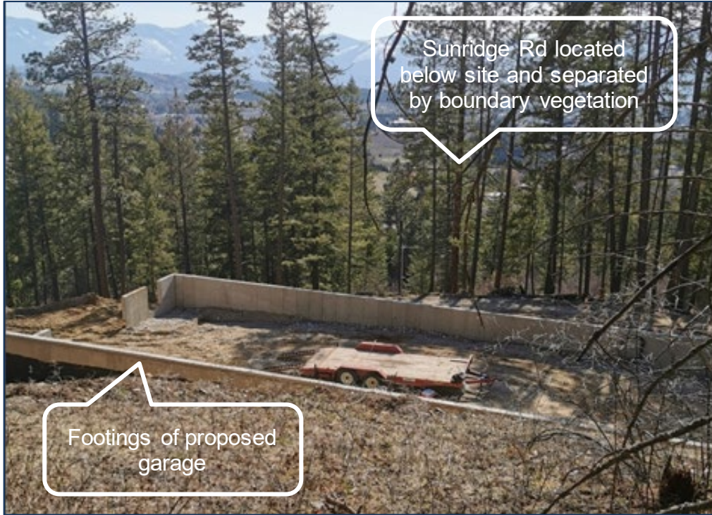
Figure 5: Location of proposed garage looking south toward Sunridge Rd. Given the topography of the site, the garage would be stepped above the access driveway and public road, and separated by retained vegetation
