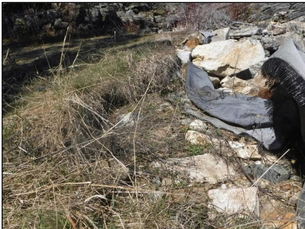
Photo 13. View of erosion along edge of terrace.
