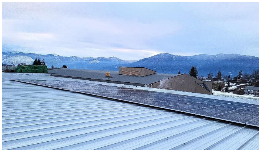
Solar array on roof of Creston & District Community Complex
