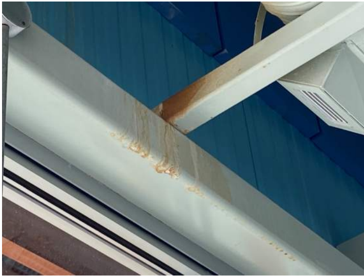
1. Interior, West Elevation Wall, far south side, white and brownish staining draining over wall panels to structural members
