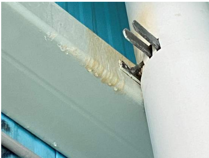
2. Interior, West Elevation Wall, south central area, adjacent to insulated drain down pipe. Active water leaking from location.
