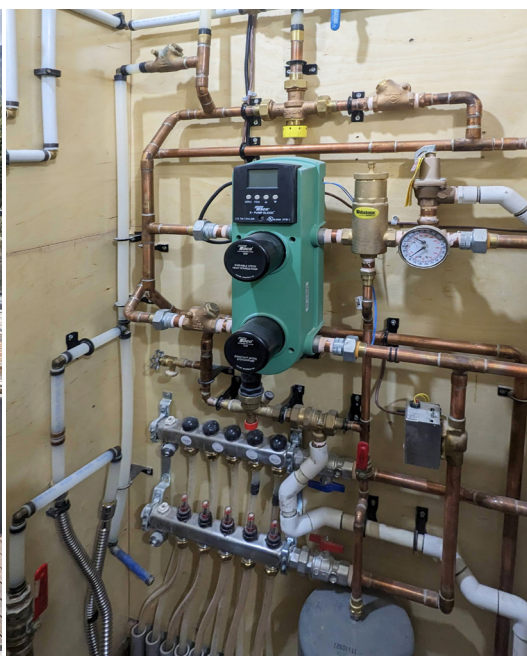
In-floor radiant heating and cooling system, supplied by the AWHP, utilizing the inherent thermal mass of the building.
