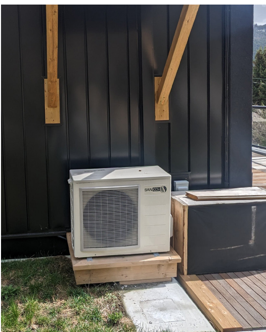
Air-to-Water heat pump (AWHP) outdoor unit providing heating and cooling to the building.
