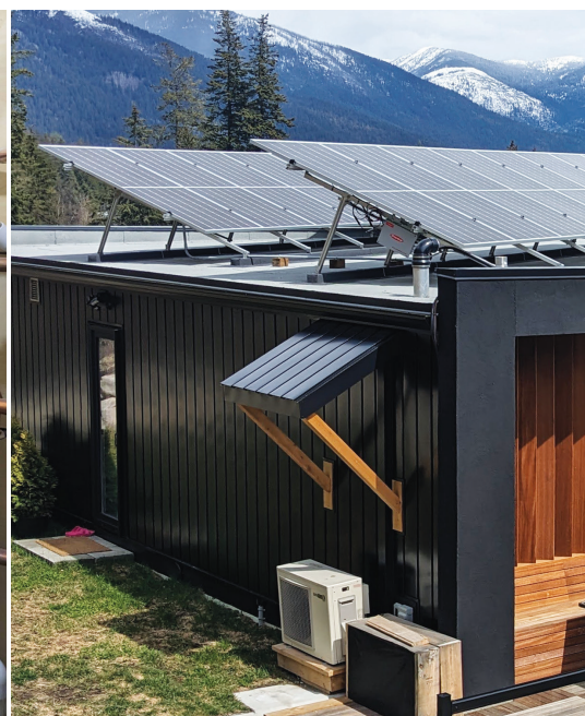
7.7 kW rooftop solar photovoltaic array connected to a grid tie-in for net metering.
